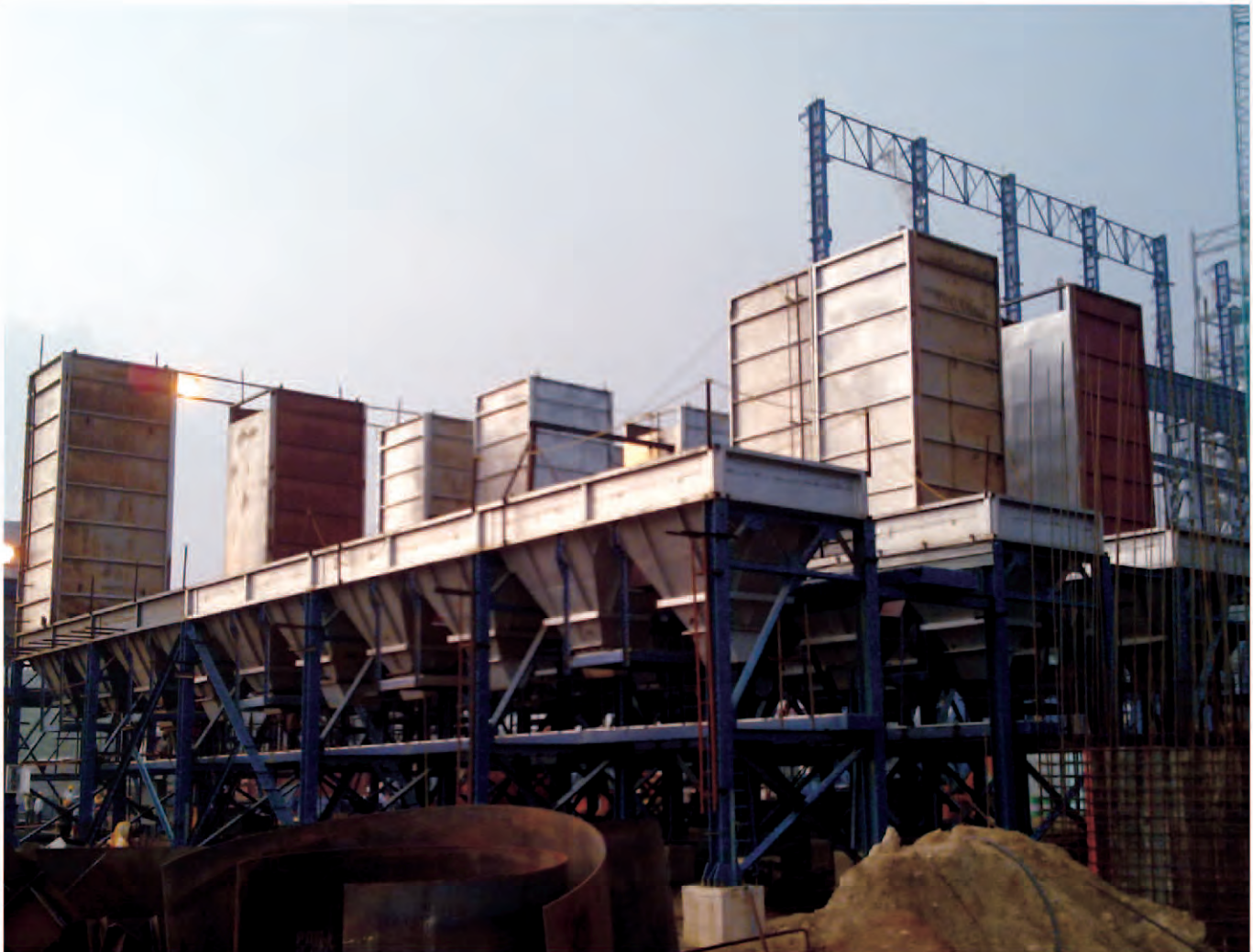
Bag House at Jindal Steel & Power Limited Angul
