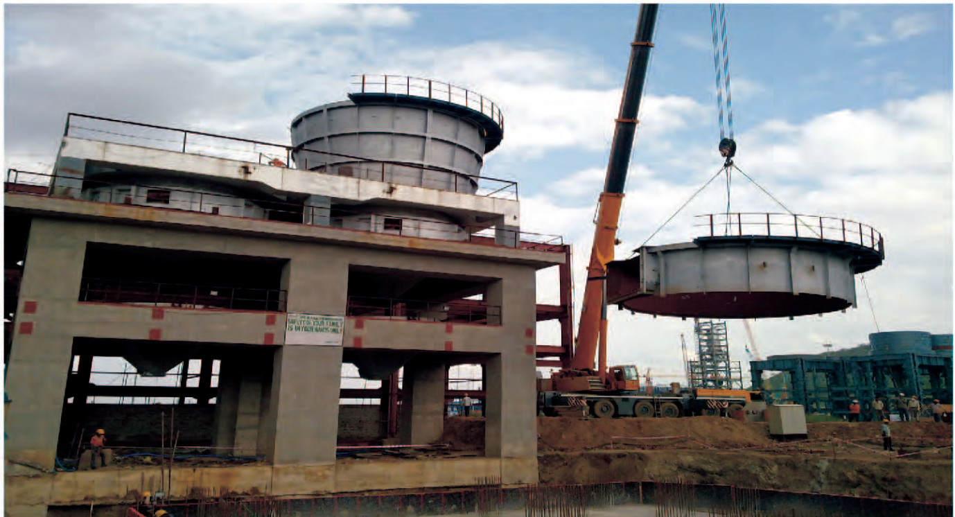
Kiln Shell Erection by 250 ton crane at Jindal Steel And Power Ltd, Angul, Orissa
