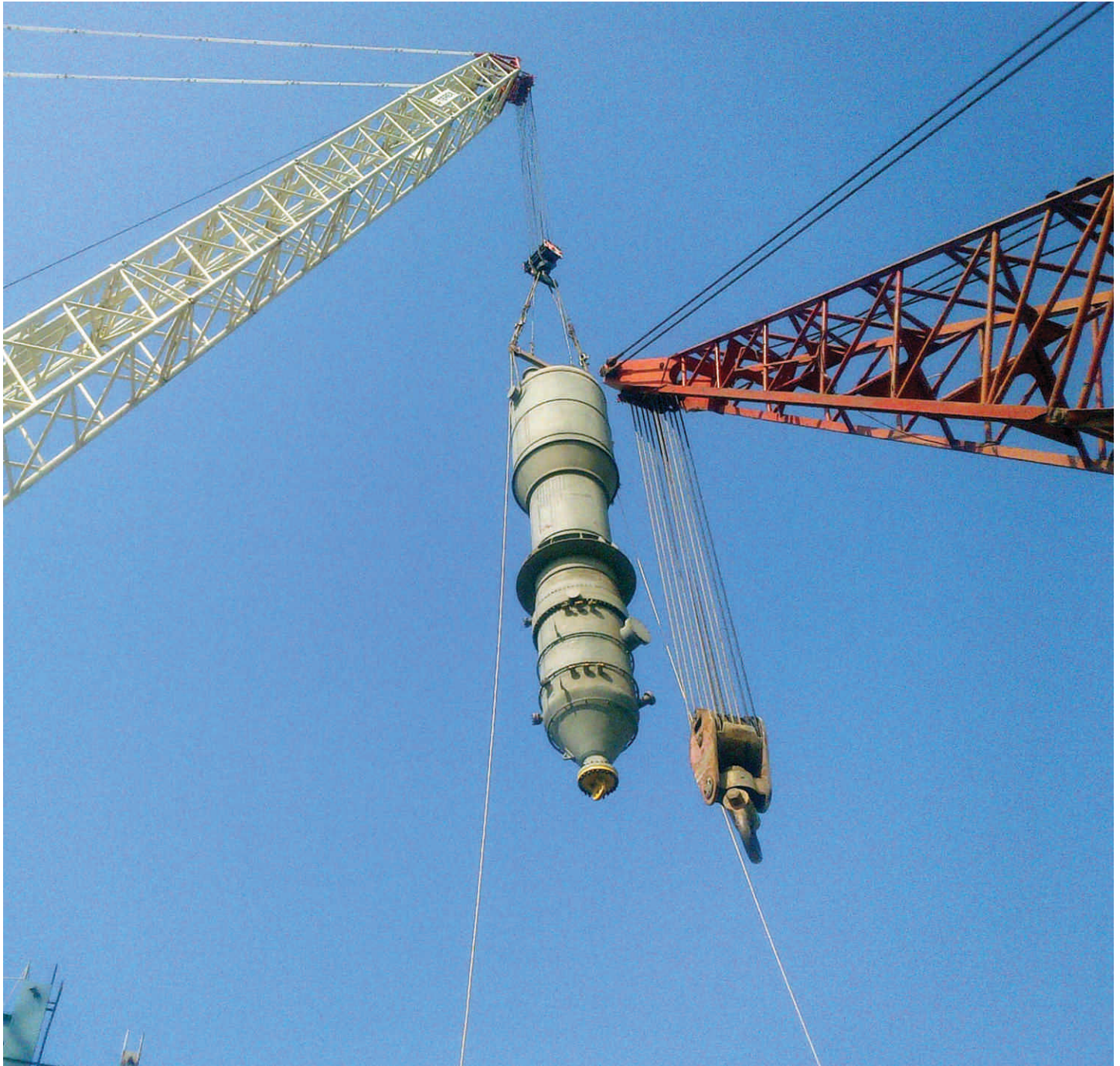
We have successfully erected 3 nos of Boiler (83 ton X 19 m long to 32 mtr elevation with a radius of 25 mtr) at Coal Gasification Plant of M/s Jindal Steel Angul with support of 450 MT crane for lifting and 250 mt crane for tailing.
