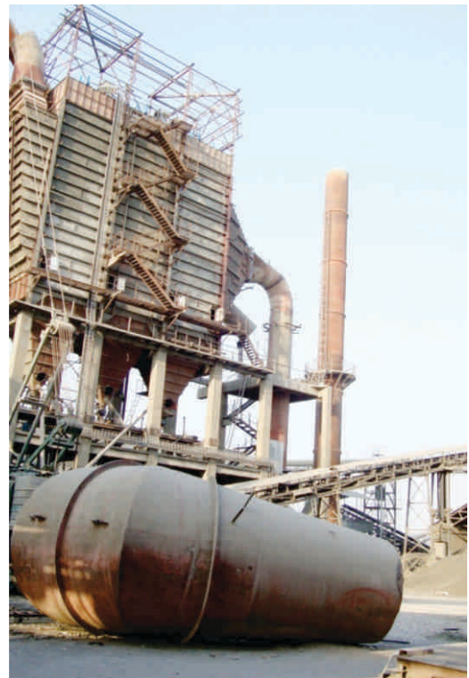
Keerthi Cements, Nalgonda Cooler ESP Outlet duct
