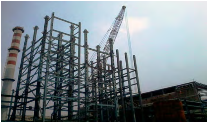
110% Achievement on Erection at Cethar Vessels Ltd, (OCL Iron & Steel Ltd), Rajgangpur in first month
