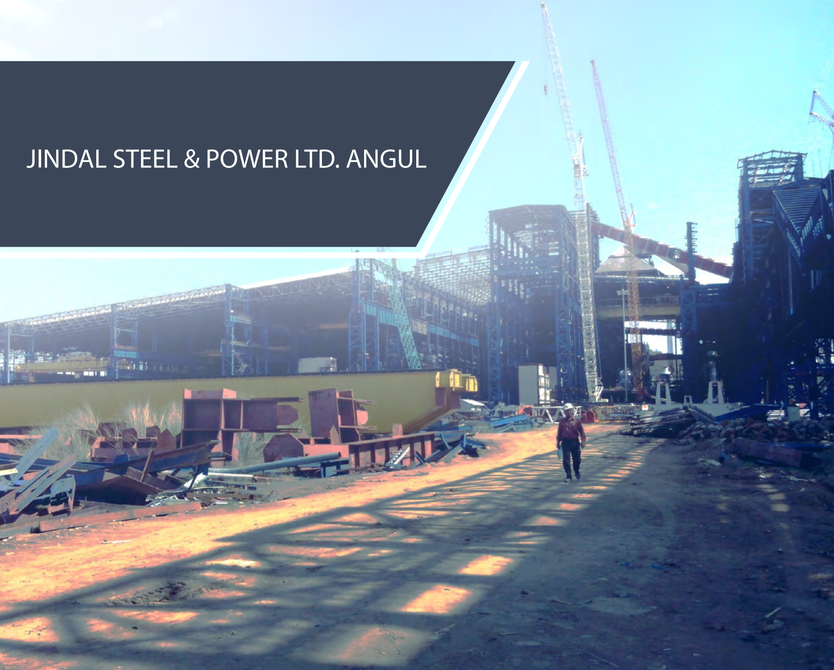
Steel melting shop & caster
