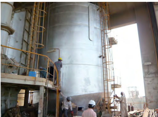
Cyclone after Erection
